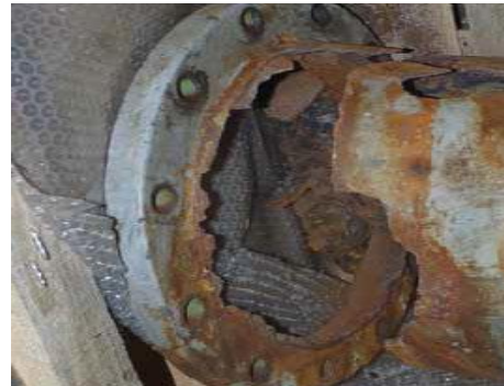
Fig. 1. Corroded piping system
