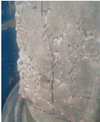
Fig. 3. Failure mode in Rattan cane reinforced Strut
